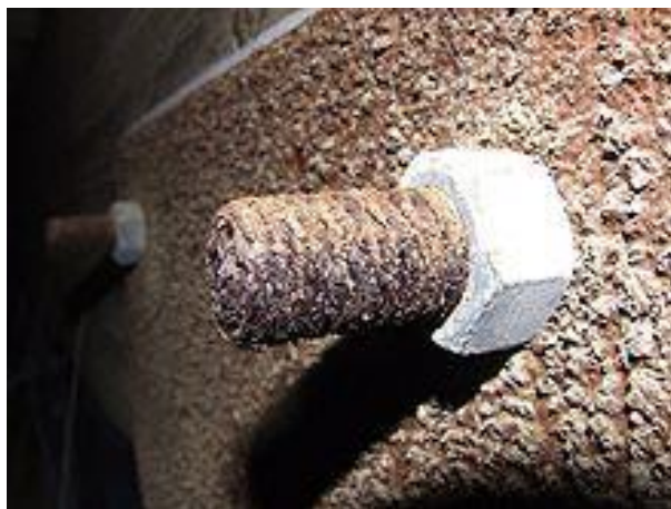
Figure 6.4.4. Corrosion on exposed metal
